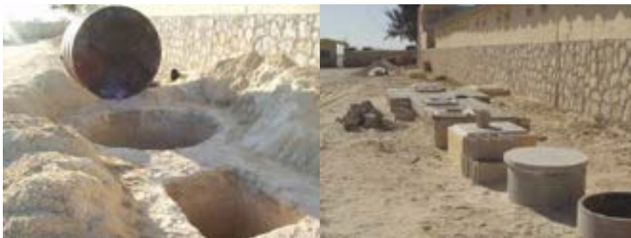
Figure 3. Waste water treatment system
