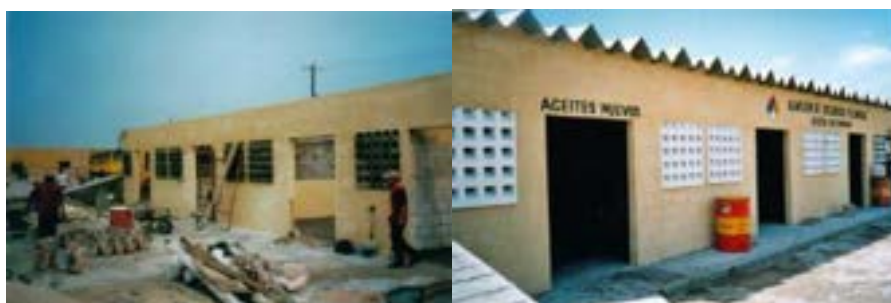
Figure 1. Change and Adjustment in the warehouse of dangerous residues
