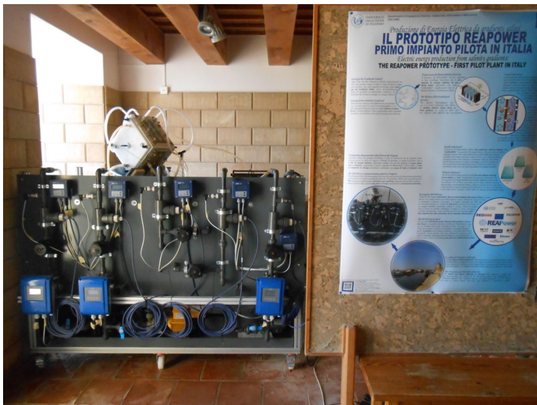
Fig. 18. View of the prototype installation, with the first operating stack equipped with 100 cell pairs of 22cmx22cm membrane area.
